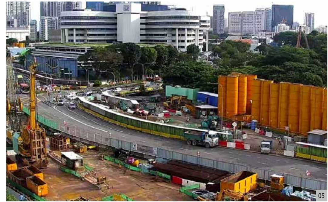
05 Singapore's North-South Corridor Sections N102 (Singapore) • Completion (expected) : 2027.04 / Client : Singapore Land Transport Authority • L=1.55km(two-way,six-lanetunnel) • An underground expressway section under construction between two MRT lines (DTL and NEL), a section considered the greatest engineering challenge among all North-South Corridor construction sites
