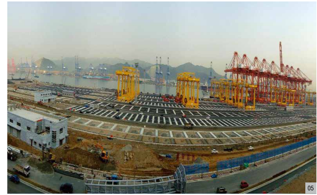
05 Electrical work of South Container Terminal (202) in the New Busan Port (Busan, Korea) • Completion : 2010.12
