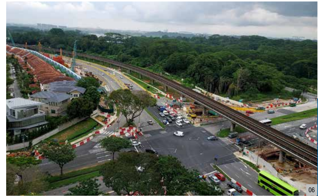
06 Singapore's North-South Corridor Sections N111 (Singapore) • Completion (expected) : 2027.04 / Client : Singapore Land Transport Authority • L=2.75km(a six-lane tunnel and overpass) • Sole contractor awarded based on the Design & Build scheme
